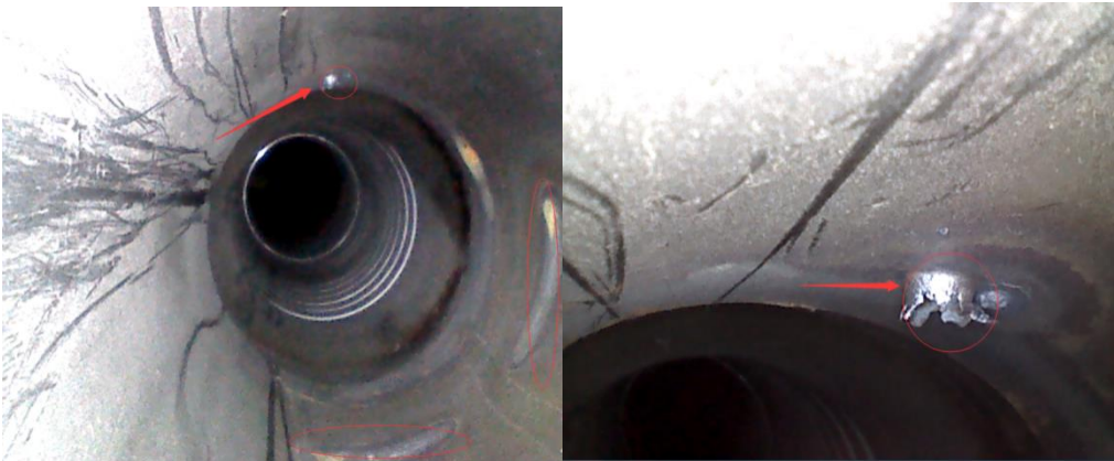
The inside flaw of the exhaust pipe
