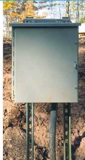
Multiple cable-drops of installed sensors can be manually accessed above grade with a tablet PC and dataPIMS™.
